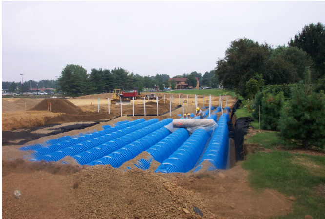
Parking lot underground storm water detention system for Walsh University
